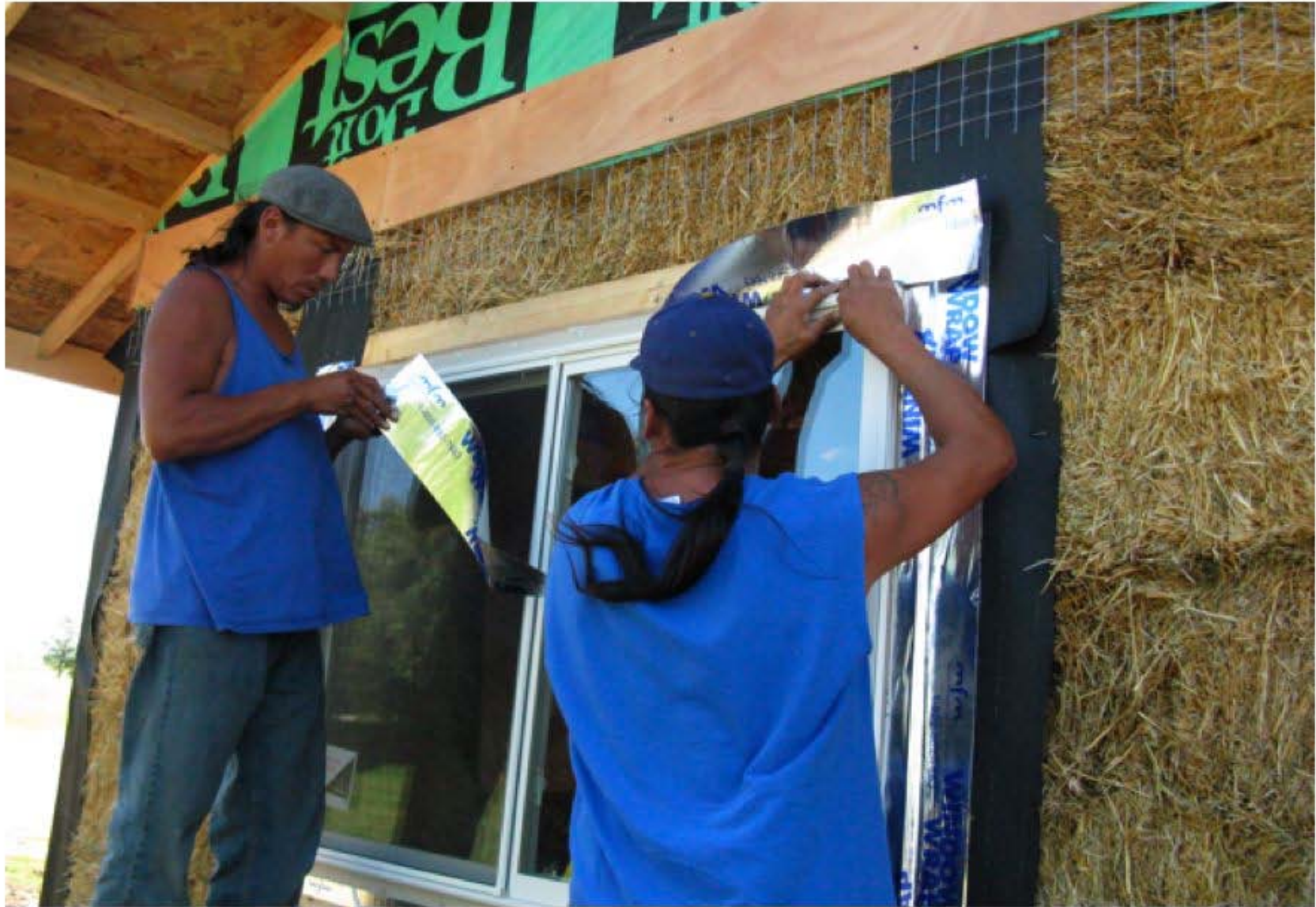
COUP SGU Buffalo Lodge Straw Bale Building Window Wrap Installation: Used to seal out water leakage along the window frame.
