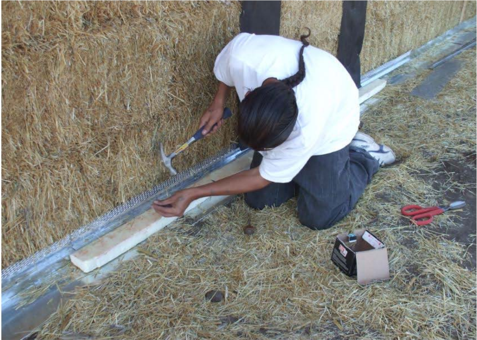
COUP SGU Buffalo Lodge Straw Bale Building Fixing J-strip for exterior plaster.
