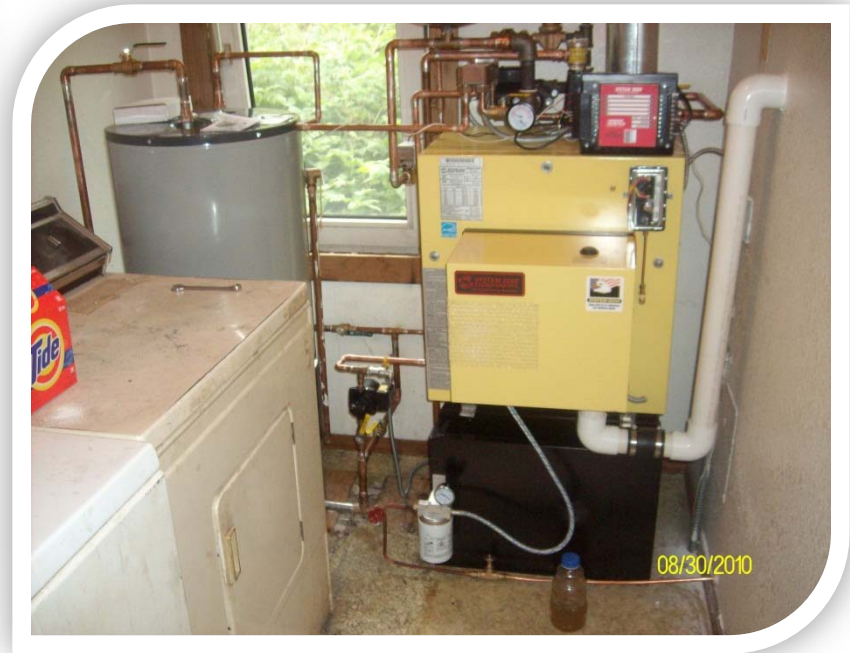
New System 2000 boiler and hot water tank
