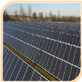
SOLAR PV FARM
